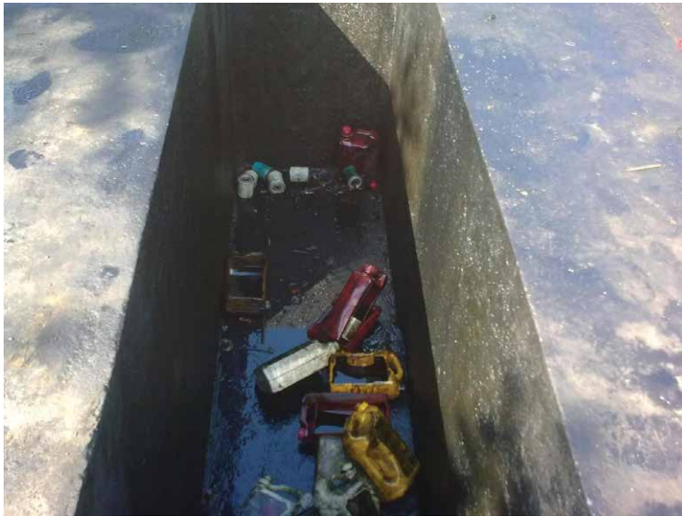
Figure 13.4: Underground Storage of Used Oil.
