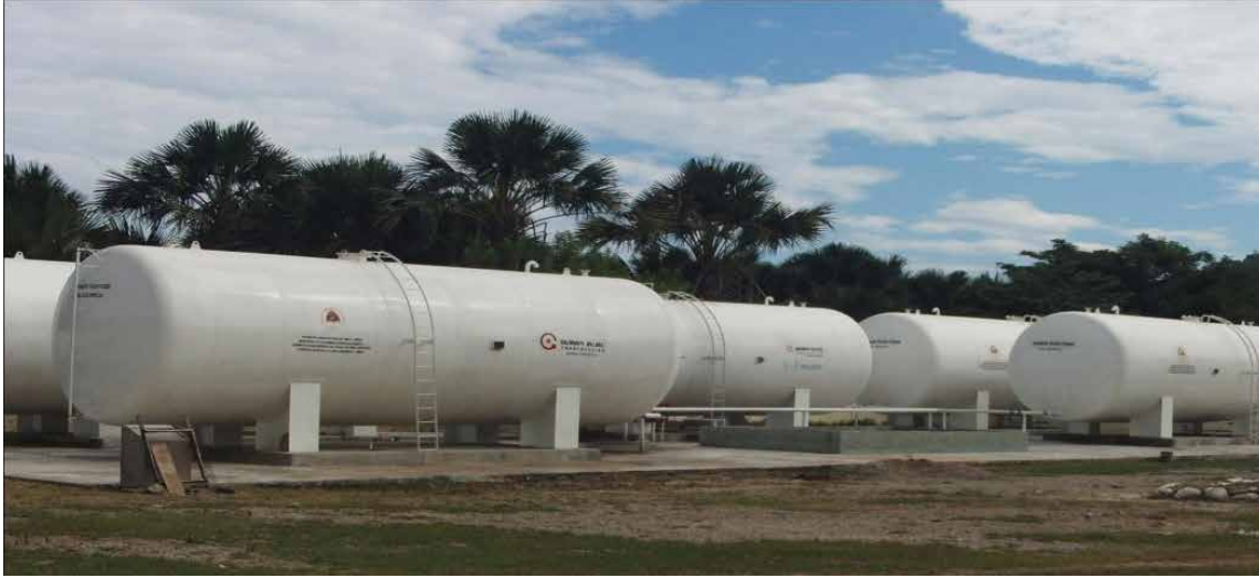
Figure 13.5: Oil Tanks Prepared by the Government.
