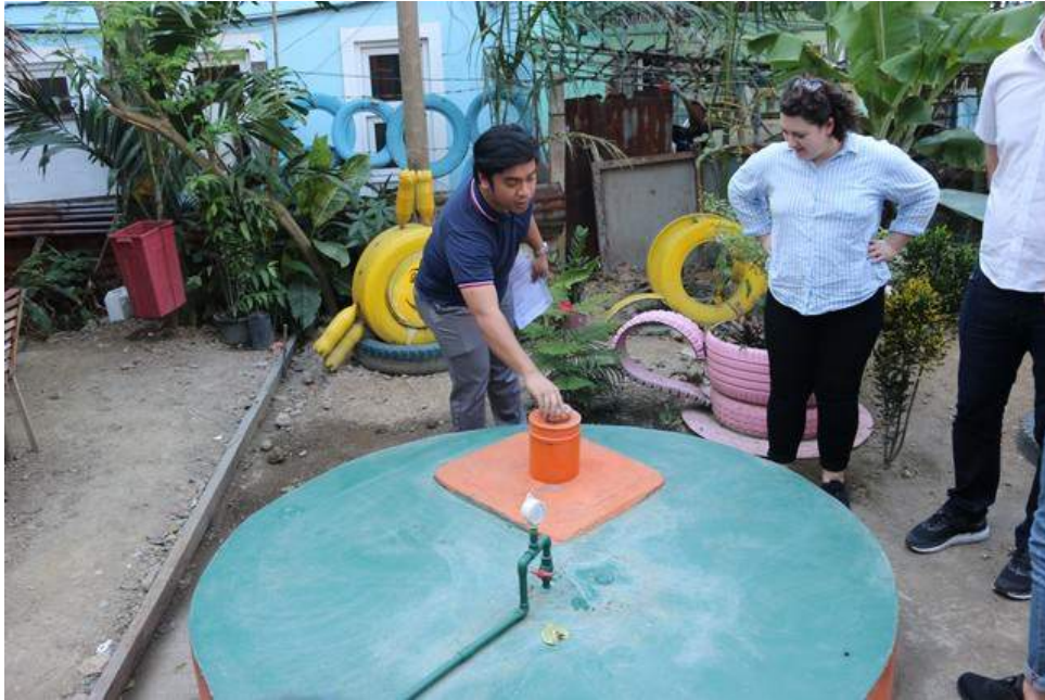
Underground biogas system, with biogas being collected through the green pipe.
